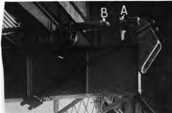
Fig. 5. Spring Bumpers on Crane and Runway. (National Tube Company.)
